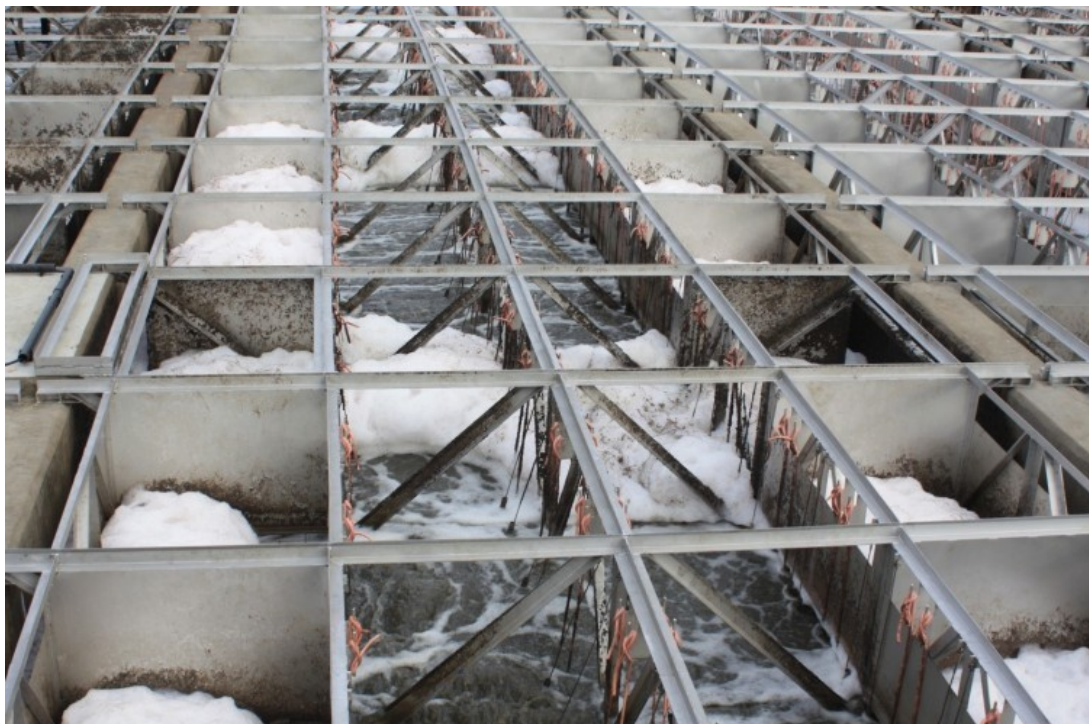
Manageable quantities of foam in reactor with Organica Biomodules installed.
