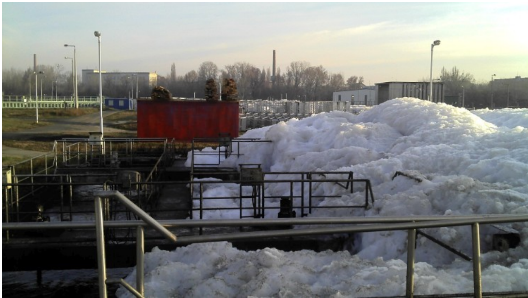
Foam overflowing from reactor with traditional activated sludge technology.
